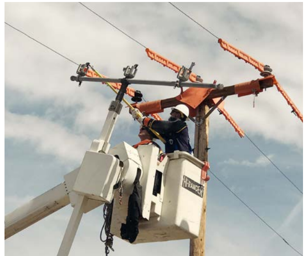
HCE Apprentice Lineman, Howard Miller (shown right), training on gloving energized lines at the Cody Hot Line School.
