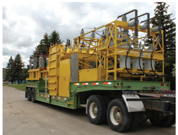
The large mobile substation waiting to go back into storage.
